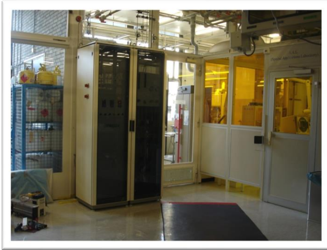
Oxygen purifier 5 Nm 3 /h – 10 Barg
