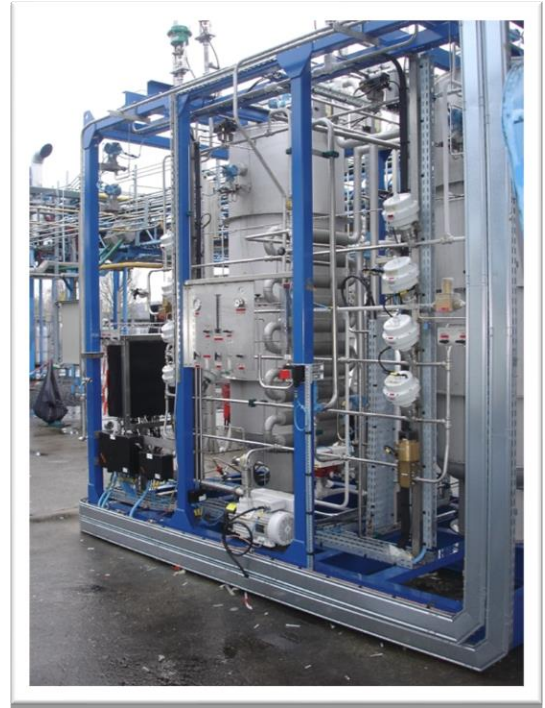
Hydrogen cryogenic Purifier 715 Nm 3 /h - 100 Barg
