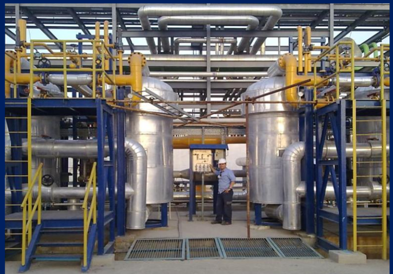
Nitrogen dryer TSA 34 000-10
