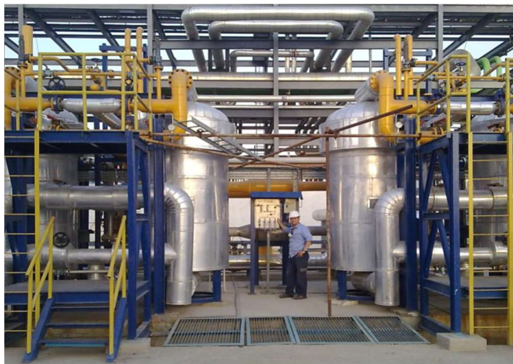
Nitrogen dryer TSA 34 000-10
