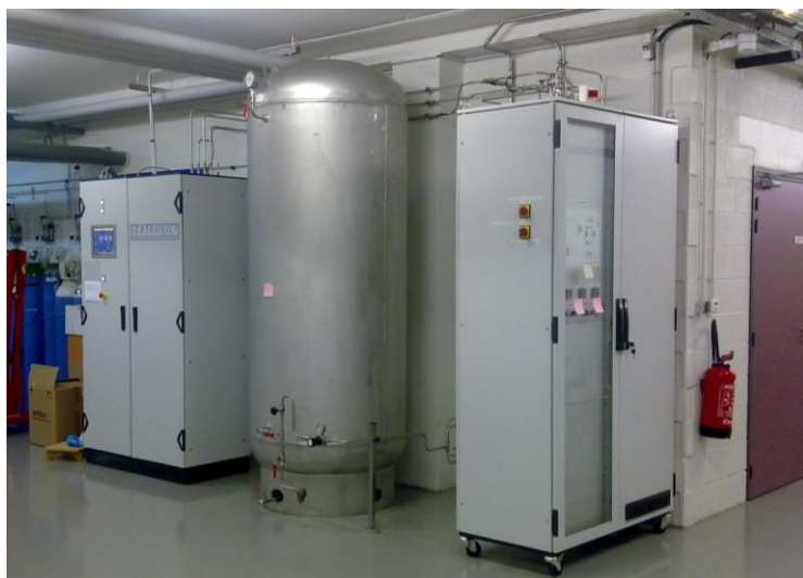
2 Air purifiers M 5-10
