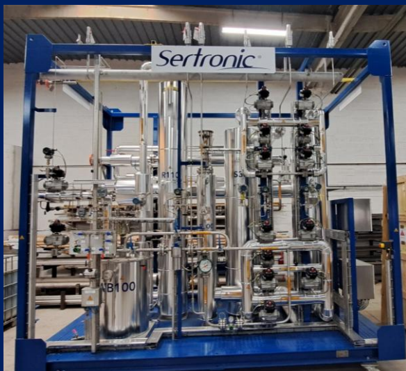
Hydrogen purification unit DS 2000-90
