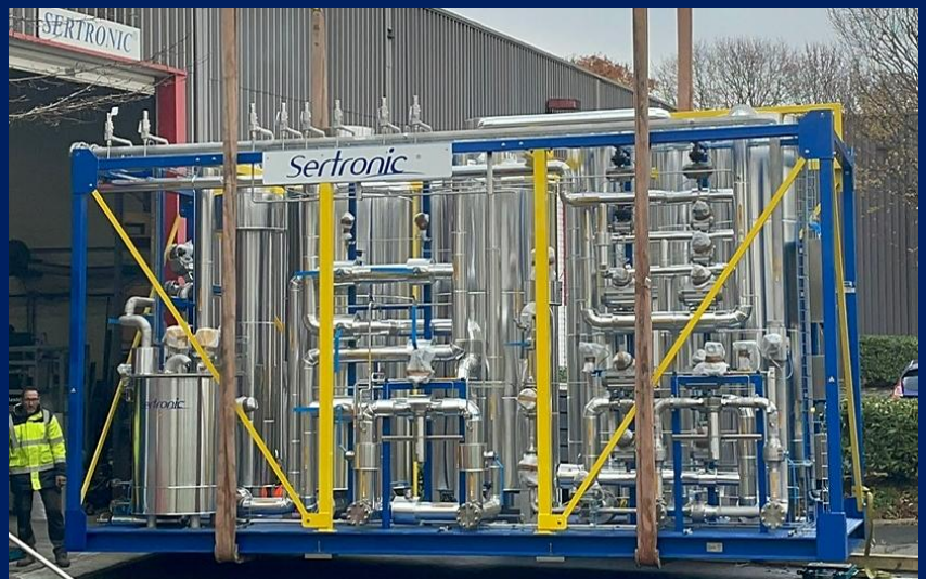
Hydrogen purification unit DS 4000-45
